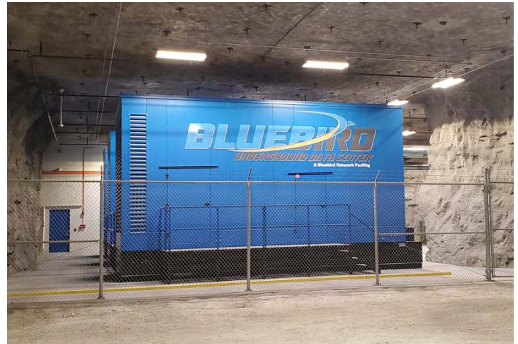
One of the three 2-MW gensets that backup the Bluebird Underground Data Center
